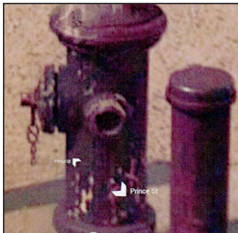
Image 4: A Google photo of a hydrant with a missing cap from many years ago was key evidence, which led to a $200,000 recovery.
