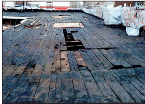
Image 3: This photo showing planks on a similar roof as the accident site was pivotal evidence, which led to a $2.5 million award.
